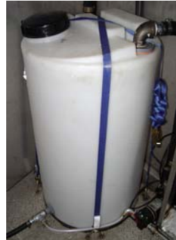
Spray Tank located inside Control Room
